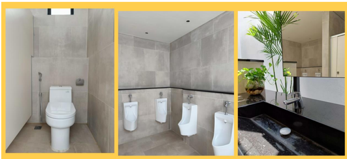
Gambar 28 Instalasi toilet hemat air Figure 28 Toilet water-efficient installation
