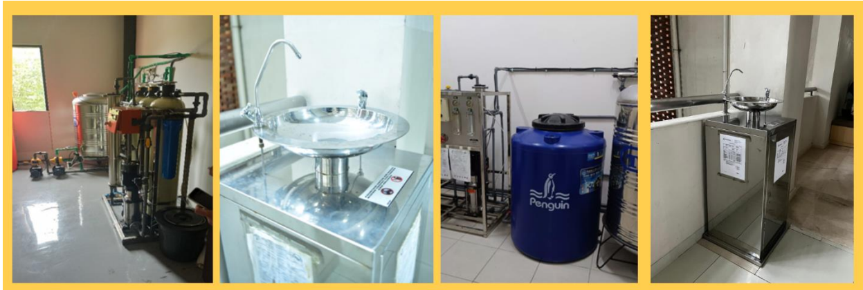
Gambar 27 Instalasi reverse osmosis Figure 27 Reverse osmosis installation
