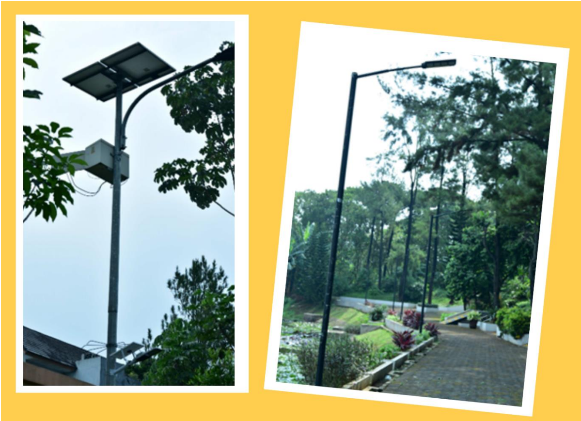
Gambar 13 Lampu tenaga surya Figure 13 Solar-powered lights
